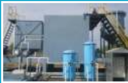
Industrial Water Treatment ETP & CETP
